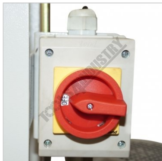
Main Power Isolation Switch
