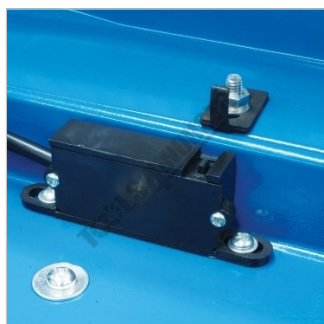
Safety Micro Switch on Pulley Guard
