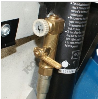
Down Feed Control
